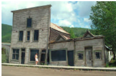
Figure 1: Dawson, AK: Abandoned Home affected by permafrost.
